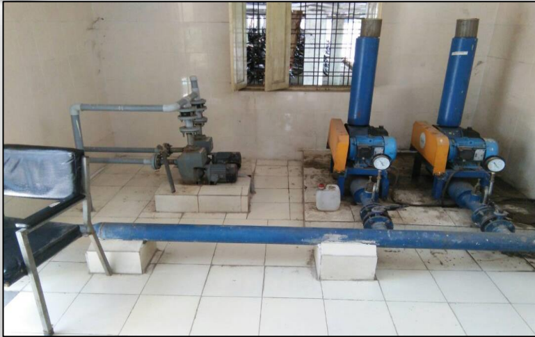
Recycling of Water & STP
