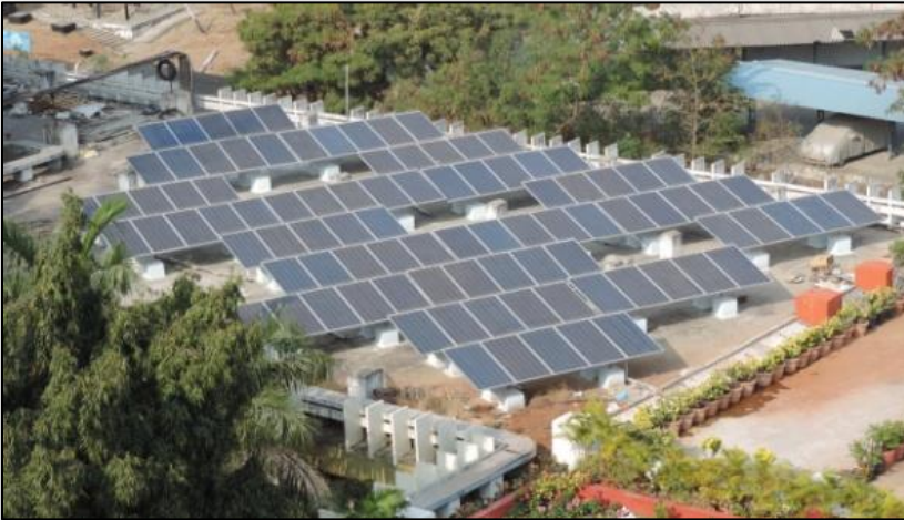
Rooftop Solar Plant
